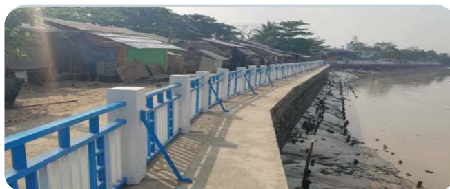
Flood protection by retaining wall in Dagon Myothit (North) Township Photo: Department of Water Resources and River Development
